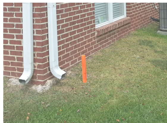
UH-1 / UH-2 INSTALLATION LOCATION WILL BE MARKED BY A STAKE AND/OR PAINT. CSPIRE/OSP WILL INSTALL CONDUIT 8" UNDERGROUND TO DESIRABLE UH-1 LOCATION.
